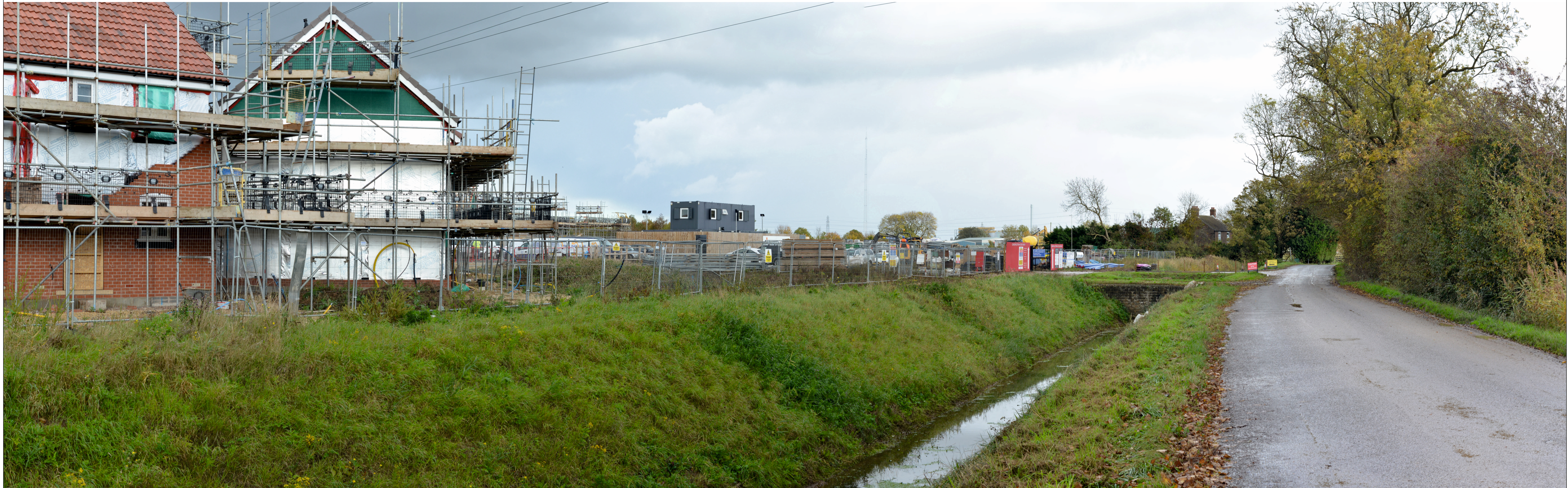
View 11: Looking east from Slippy Gowt Lane alongside properties off Wyberton Low Road (near Sustrans Route 1 / North Sea Cycle Route)
